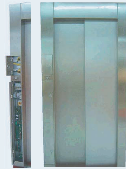
Controller in door frame
