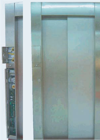
Controller in door frame
